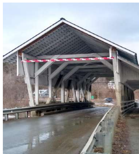
Millers Run Bridge with reflector tape – by Jeanne Beaudry
