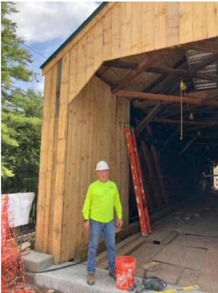
Pictured is Jim Ligon standing at east portal of the nearly finished Kingsley covered bridge. Photo by Beth Brown Limmer
