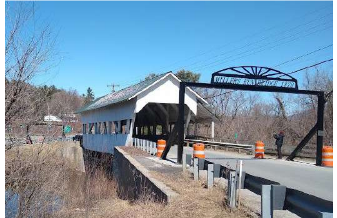
Miller's Run Covered Bridge new headache bars - Photo by Jeanne and Marcel Beaudry
