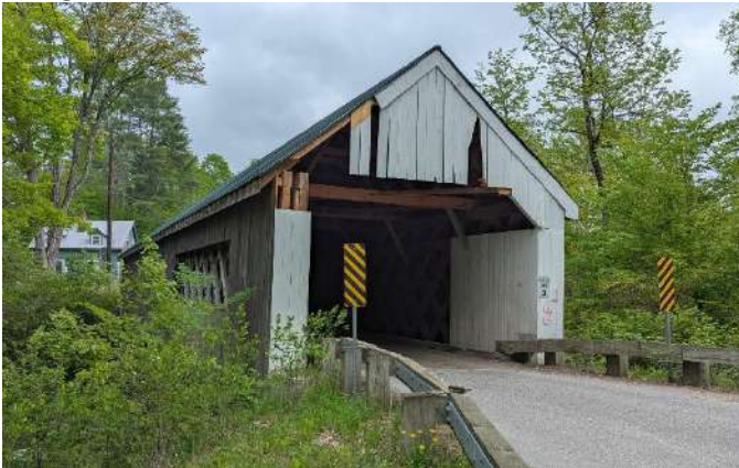
Damage to Williamsville Covered Bridge - Photo by Bill Caswell
