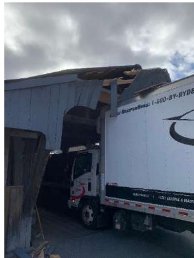
Truck stuck at a covered bridge in Waitsfield, Vt. – Photo courtesy Miles Jenness
