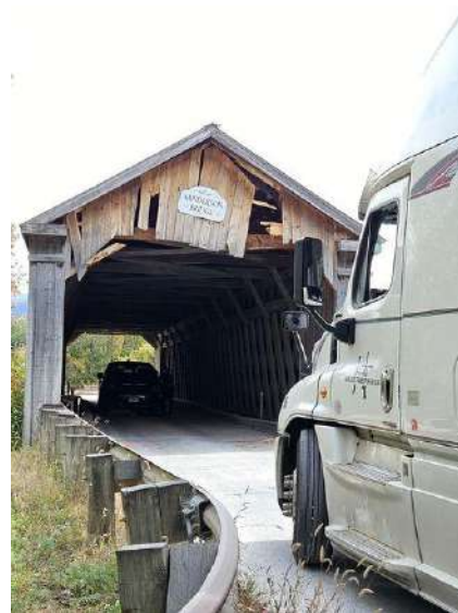
Sanderson damage 10-4-24 Photo Courtesy Paul Limmer
