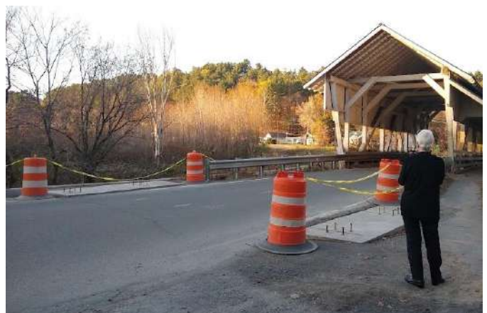
Jeanne Beaudry surveying new footings for steel beams at Millers Run CB - photo by Marcel Beaudry
